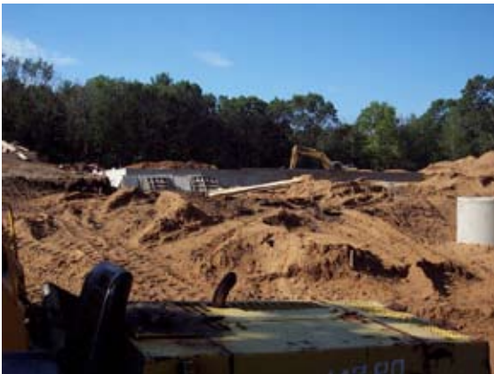
The next day soil was filled in over the tubes , leaving only the vertical intake tube visible (at right)
